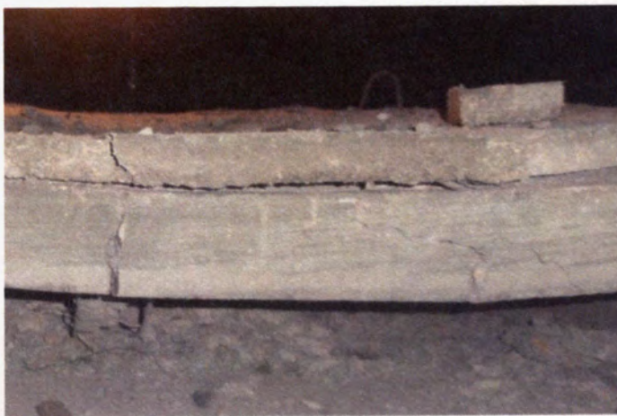
(e) Flexural Cracks in the Back Face
