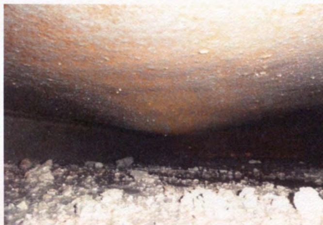
(e) Bulge in Tension Face
