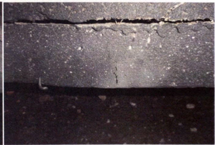
(f) Crack and Delamination Front Face
