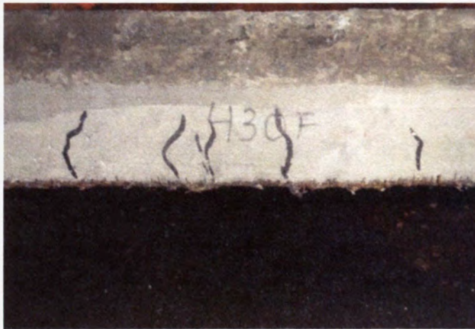
(c) Flexural Cracking in the Front Face
