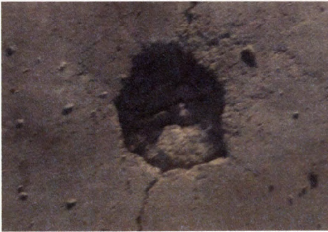
(c) Punching Failure
