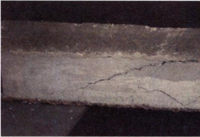
(c) Shear Crack in the Front Face
