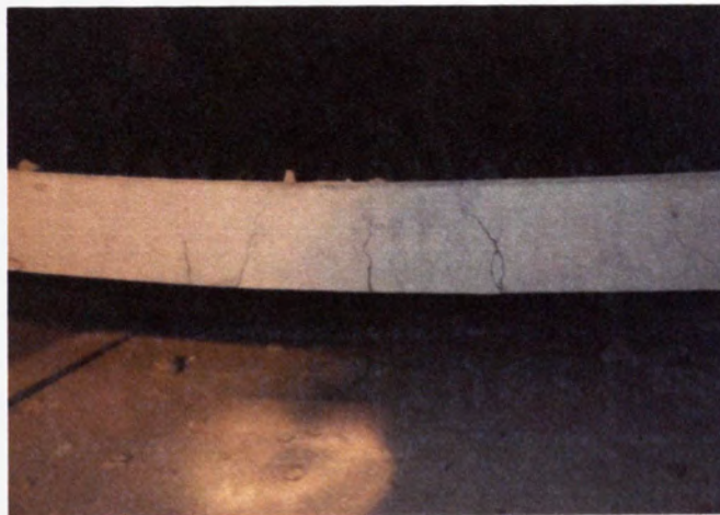
(c) Flexural Cracks in the Front Face
