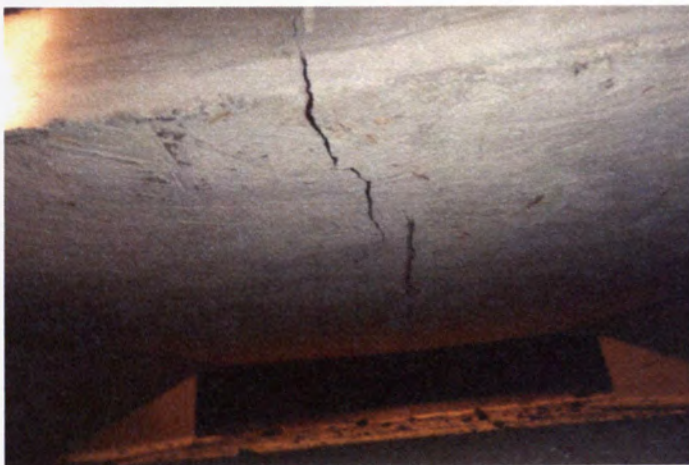
(c) Flexural Crack in the Tension Face
