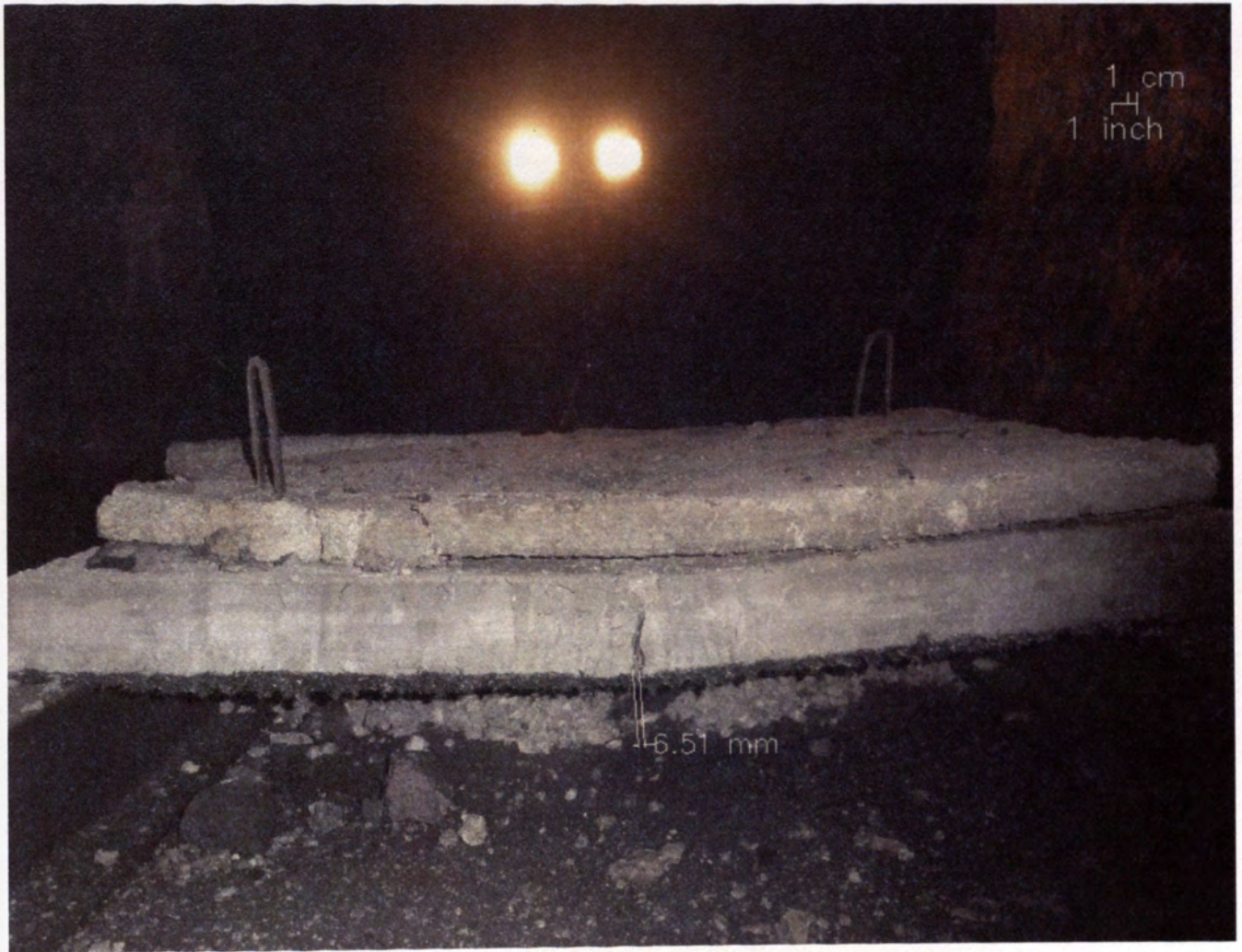
Figure E.12 – Flexural Cracks in the Back Face of H-A/F, 2 nd Event
