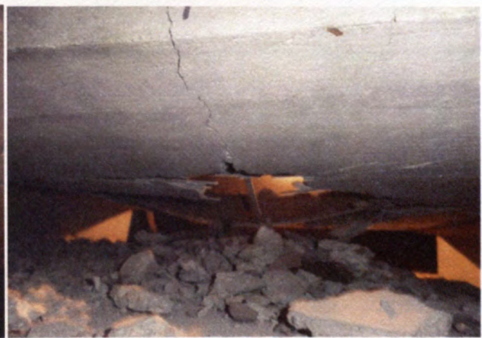
(f) Debris and Tension Face
