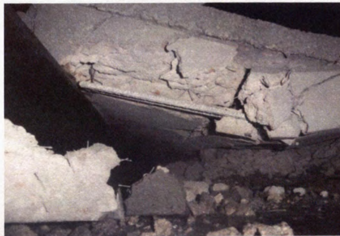
(e) Crack and Debris From Front
