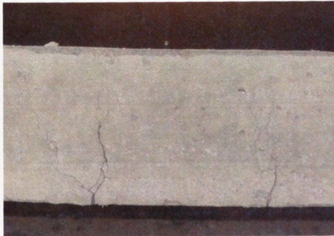
(c) Flexural Cracks on Back Face
