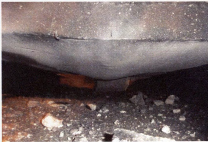
(c) Large Bulge in Tension Face
