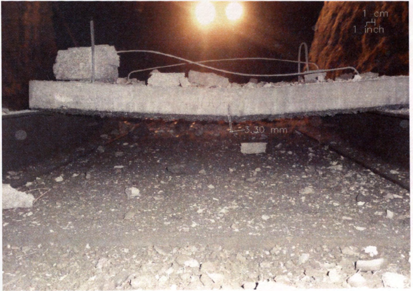
Figure E.13 – Flexural Cracks in the Back Face of H-FG-A/F, 2 nd Event
