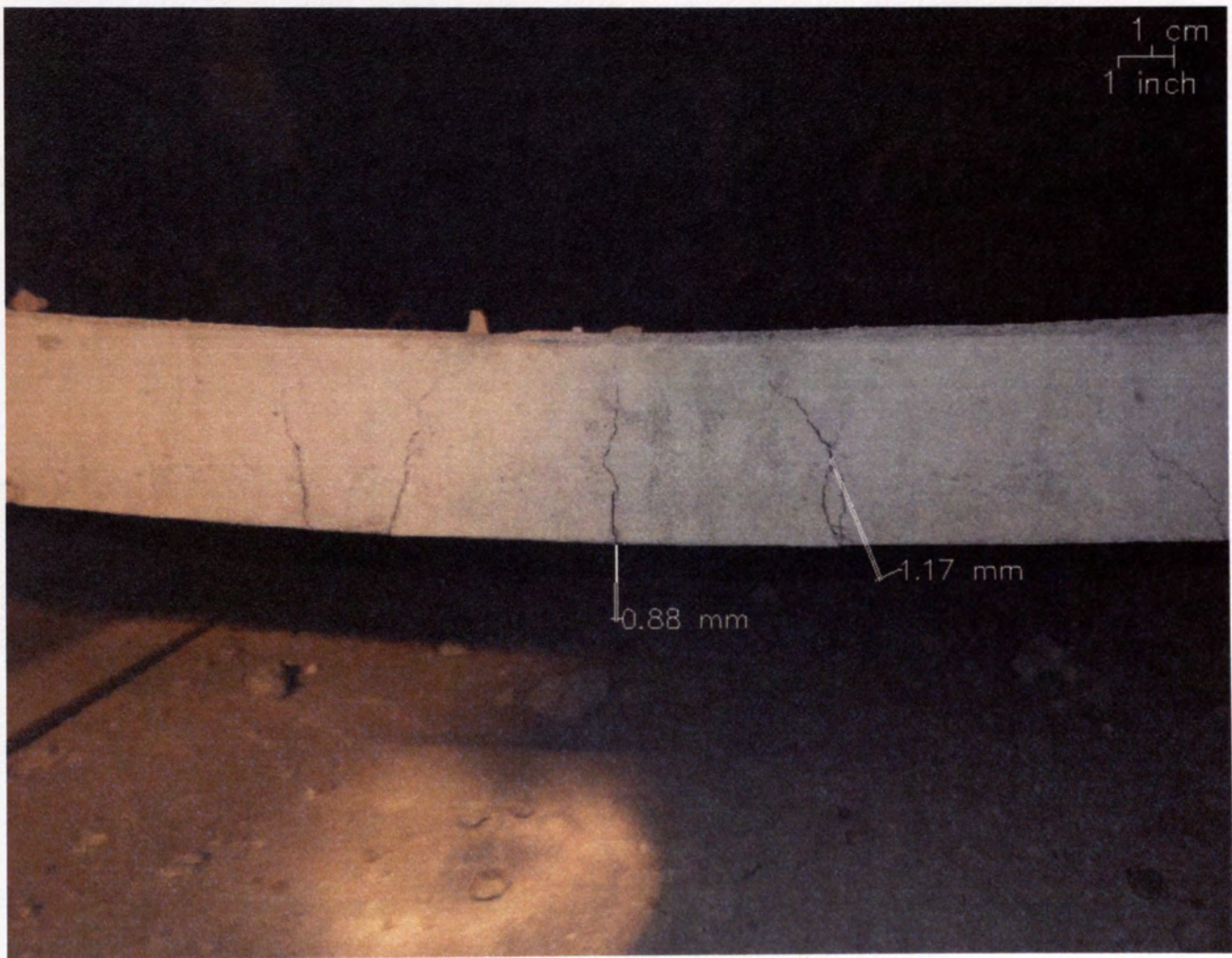
Figure E.5 – Flexural Cracks in the Front Face of 2-RC
